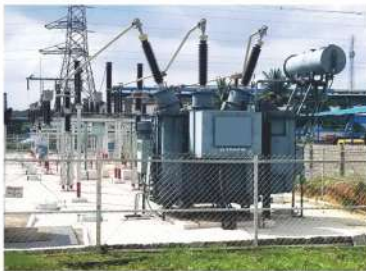
Distribution Transformer with Detachable fins
